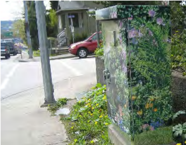
Creative camouflage of an above ground utility vault.
